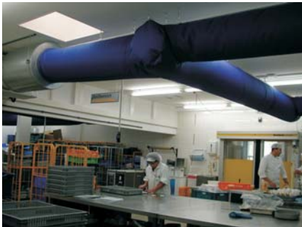
1. Textile air distribution in the kitchen
