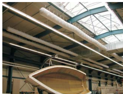
2. Installation with insufficiently tightened wire
